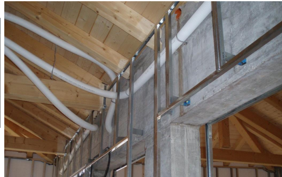
Mechanical ventilation system
