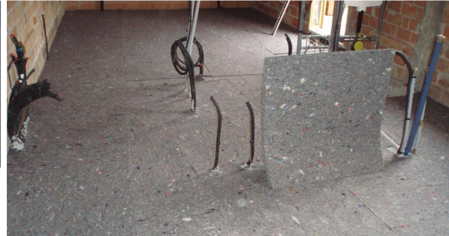
Photovoltaic system - TNT underflooring above systems
