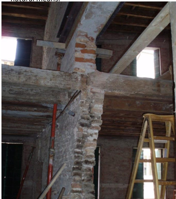
Crooked walls, before renovation
