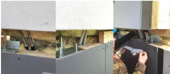
Figure 6. HVAC connections between the modules (11 a.m.)
