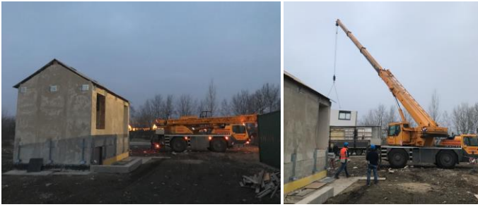
Figure 4. Installation: 6 a.m.: Prepared anchors on the simulated original building's façade. Unloading the first modules
