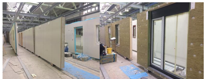
Figure 3. Prefabricated modules in the RD Rýmařov factory before finishing the final plaster layers
